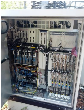
base station cabinet
