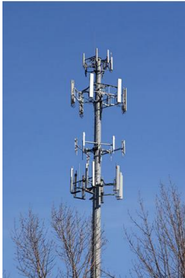
base station tower
